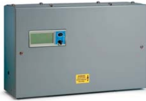
EBMMPCT250 250A multi-function (Located below Type B Distribution board)
